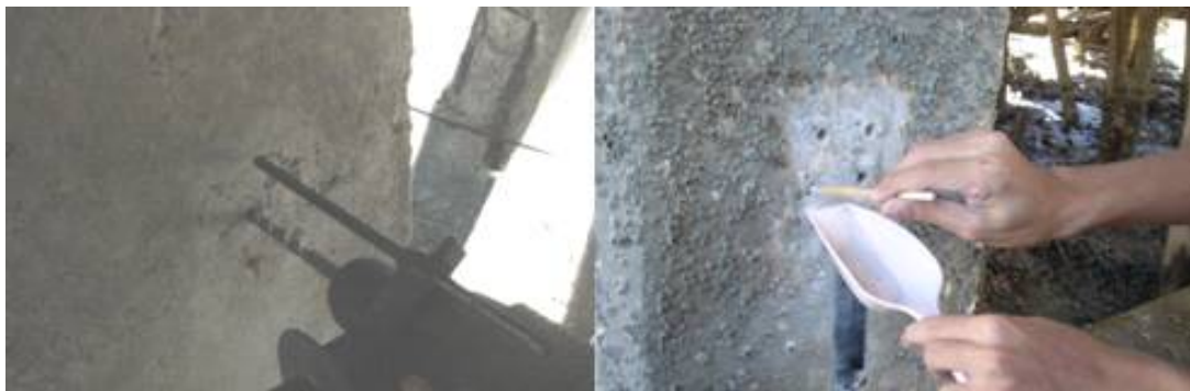
Figure 31 Drill concrete at depth level that is wanted then save the powder example
