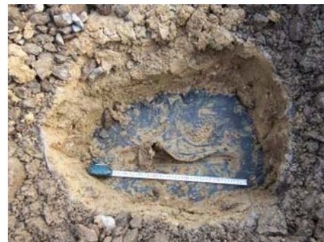
Figure 2. The defect in geomembrane
