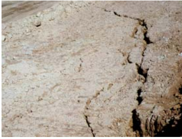
Figure 4a Crack in embankment
