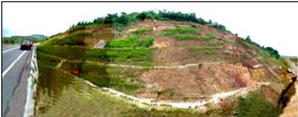
Figure 18a Overview of cut slope failure
