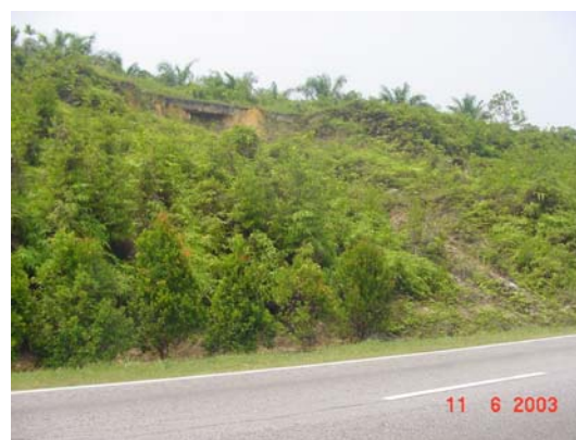
Figure 15a View of slope failure
