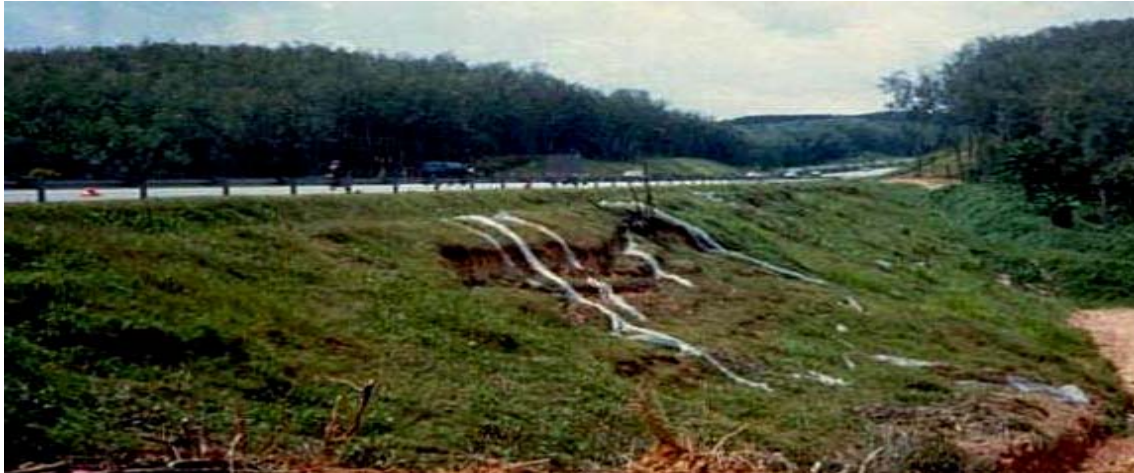
Figure 10a Picture of embankment failure, 1989.
