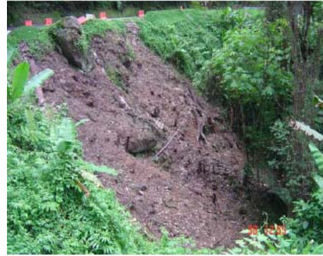
Figure 19a Collapse of embankment
