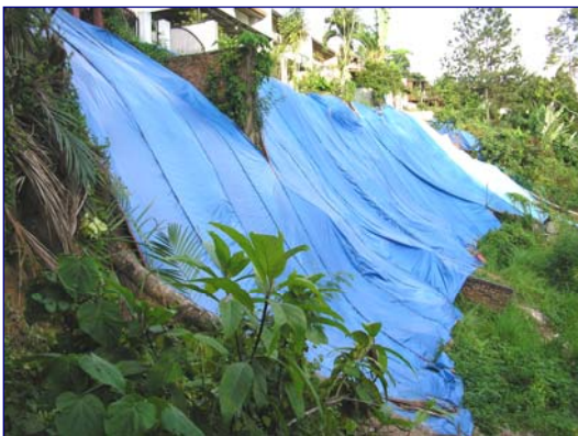
Figure 20a Condition of Zooview slope in 2004
