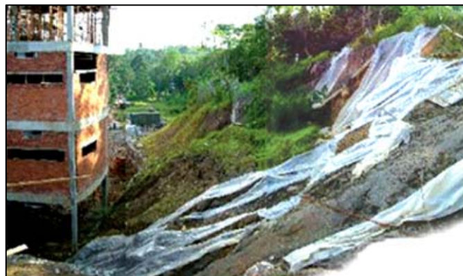
Figure 16a Slope failure affecting the lecture block
