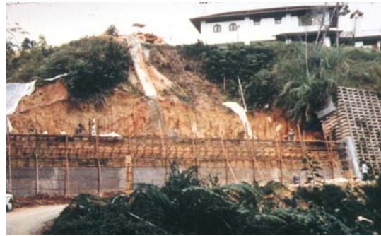
Figure 2a Petronas bungalow with failed slope in 1987
