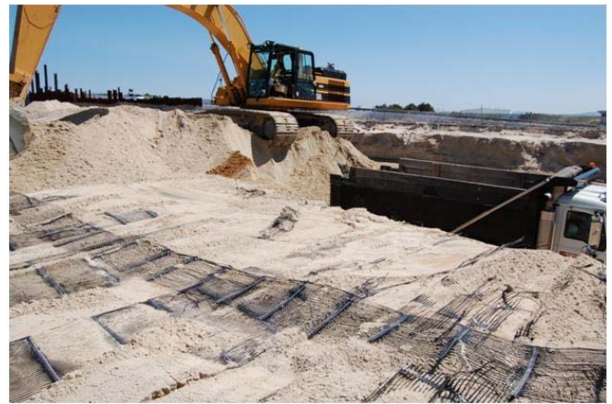
Figure 6. Excavator on top of unreinforced steep sand slope
