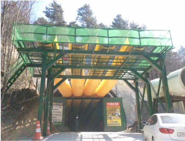
Figure 36 Ventilation tubes for construction (110 KW)
