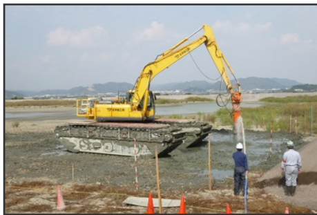
Photo 4 Situation that the ground is being mixed by agitator-attached excavator with addition of water
