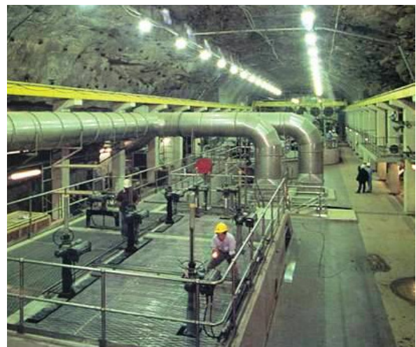
Figure 4 Sewage treatment works at Stanley, Hong Kong
