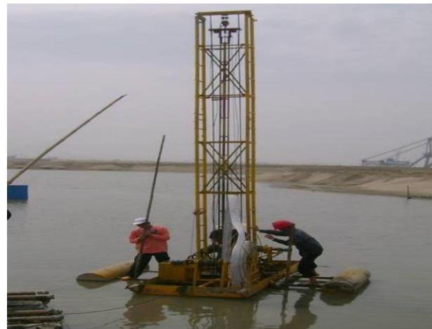
Figure 18 Floating vertical drain installation rig for installation of short drains (Courtesy of Yan S.W.)
