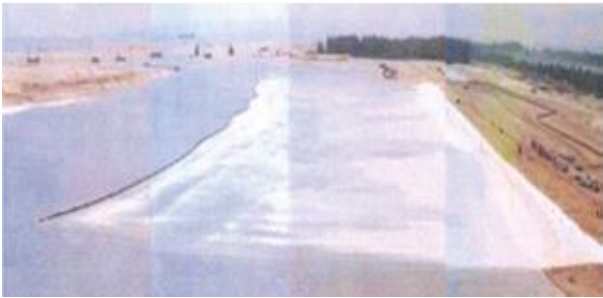
Figure 15 Installation of geotextile sheet for the slurry pond land reclamation project in Singapore (after Chu et al. 2009a)
