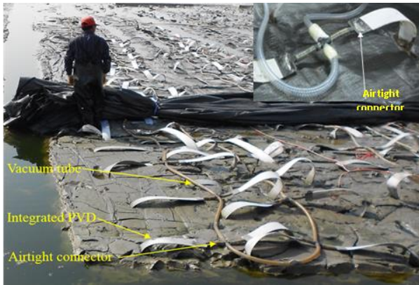
Figure 19 Connectors used to connect PVDs directly to the vacuum distribution pipes (after Wang et al. 2016)
