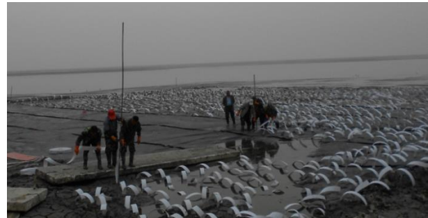
Figure 17 Installation of PVDs from a platform made of foam boards (after Wang et al. 2016)
