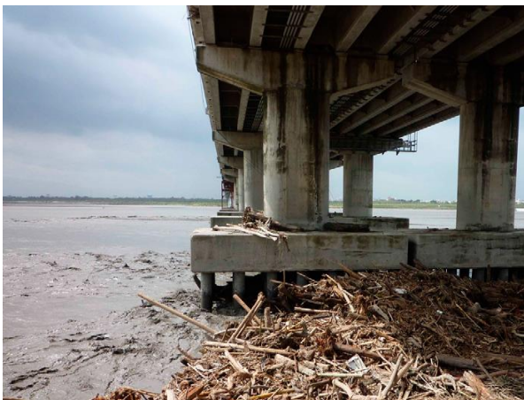
Figure 1 A highway bridge threatened by scour and debris during 2009 Typhoon Morakot (Lee et al, 2010)
