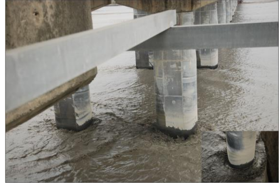
Figure 7 Scour occurring to Pier 42 during Typhoon Morakot
