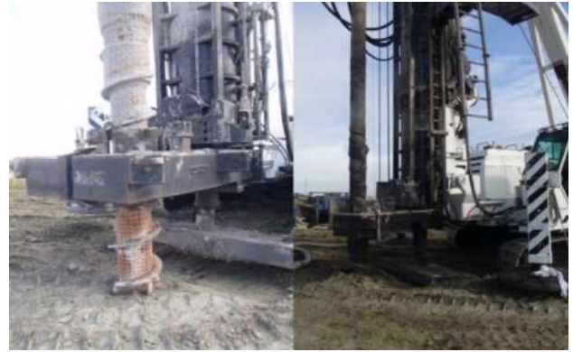
Figure 10 Omega pile installation, test pile instrumented on the reinforcement cage at 6 depth locations.
