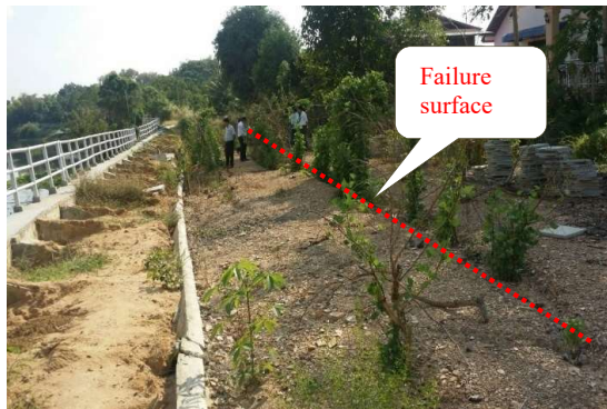
Figure 3 Failure surface in plan (lateral moment)
