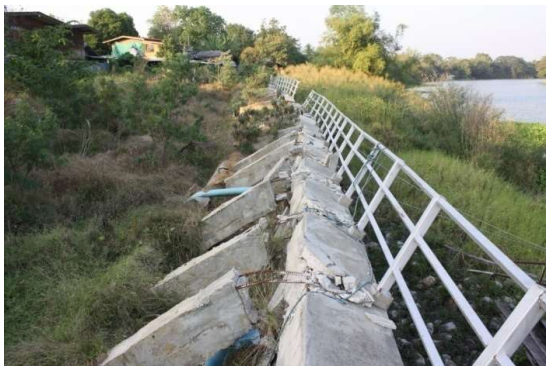
Figure 4 Damages to existing retaining wall
