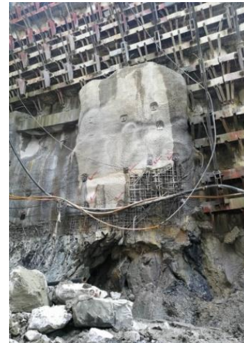
Figure 8 Figure of exposed rock face around which some of the anchors had experienced loosening
