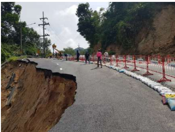
Figure 5 Road damage due to Kratu-Patong 2022 landslide in Phuket
