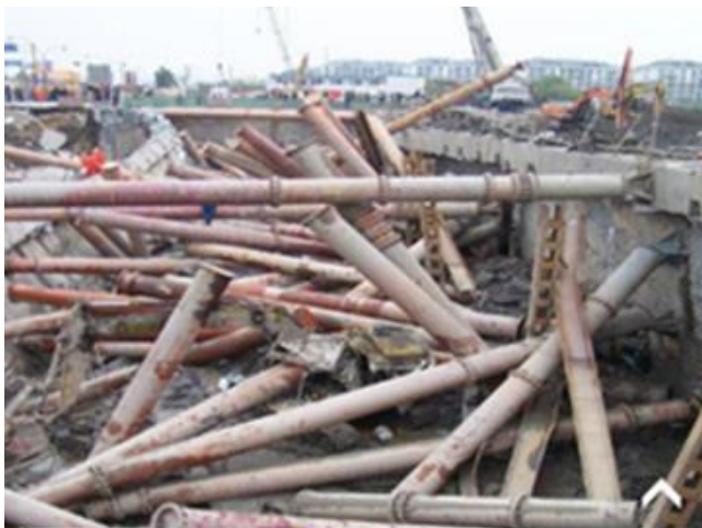
Figure 2 Failure of excavation (source: internet)
