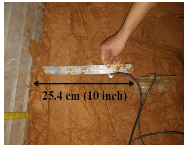
Figure 9 The pore pressure sensor (P2) at the desired location
