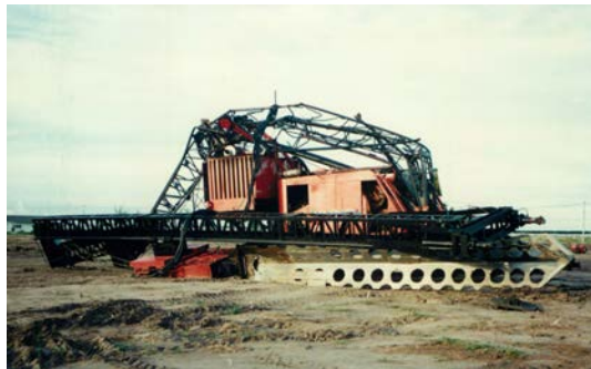
Figure 5 The collapse of a compaction rig because of extracting the probe at the resonance frequency
