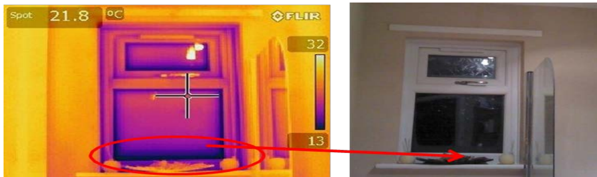
Figure 21: Detections around windows at the bottom.
