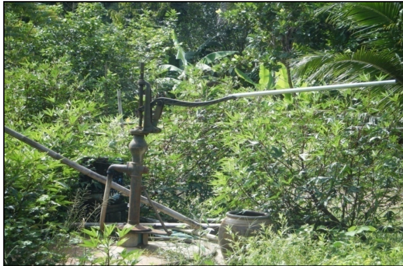
Figure 44 An artesian well from the Office of Accelerated Rural Development (ARD) established in the north of BTS.
