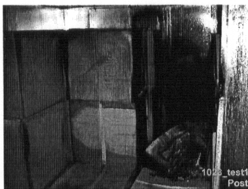
Appendix Figure B11 Post Fire Test in LD3 Containers Removed Revealing Damage
