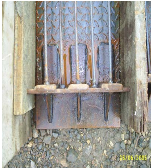
Appendix Figure C3 Reinforcement at the end of specimen
