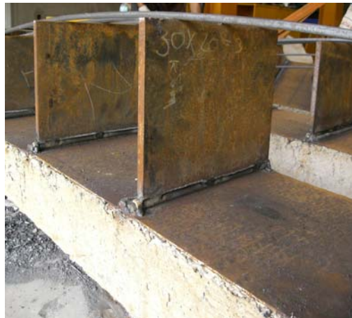
Figure 41 The joint at transferred plate to checkered plate changed as hinge joint for the re-test in actual test.
