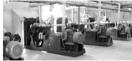
Biogas generator sets, Veerachai Farm
