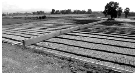
Final effluent solids drying bed, SPM Feedmill Farm
