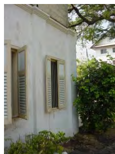
Figure 152 & 153: Typical bearing wall for government building, tobacco company in Chiang Mai, (taken by Vitul L., 1/2/02)
