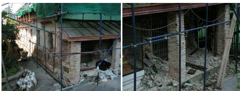
Figure 211 & 212: Repairing of brickwork by re- plastering in Wat Phra That Chaehang, Prae (taken by Vitul L., 2/4/06)
