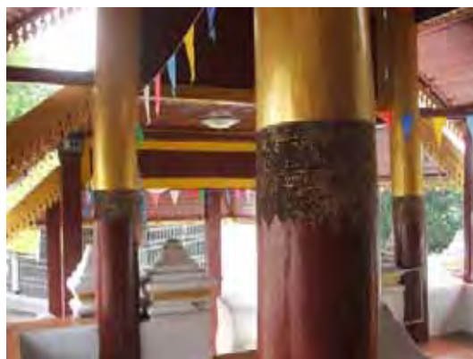
Figure 212: Remains of original decorative pattern on the pillars. (Photograph: 07.11.2008)
