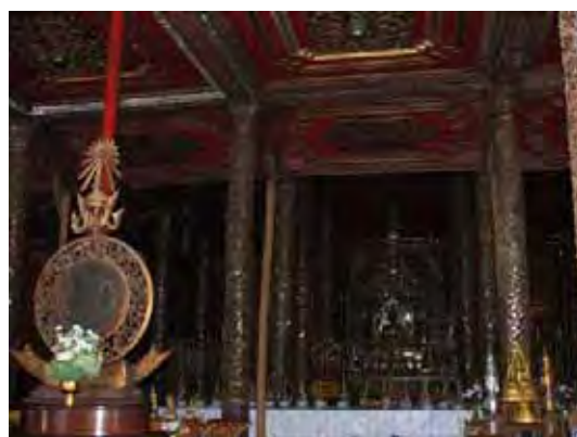
Figure 177: Condition of interior of the monastery. (Photograph: 17.11.2008)
