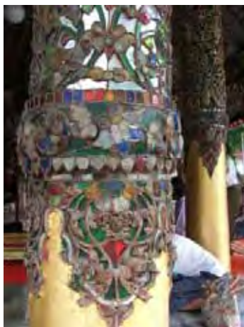
Figure 164: Missing colored glass.
