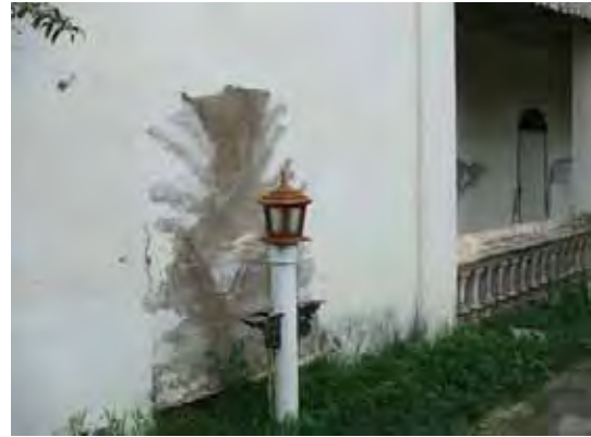
Figure 198: Efflorescence effect according to ground water.
