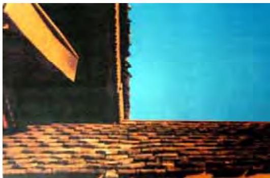
Figure 209: Condition of the traditional clay roof tiles before restoration by Fine Arts Department. (Source: Fine Arts Department, 07.07.2009)
