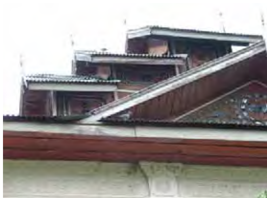
Figure 195: Condition of the upper part of monastery.
