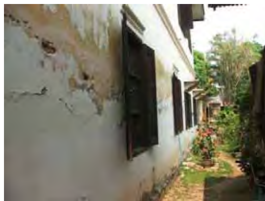
Figure 237: Trace of flood and underground water.
