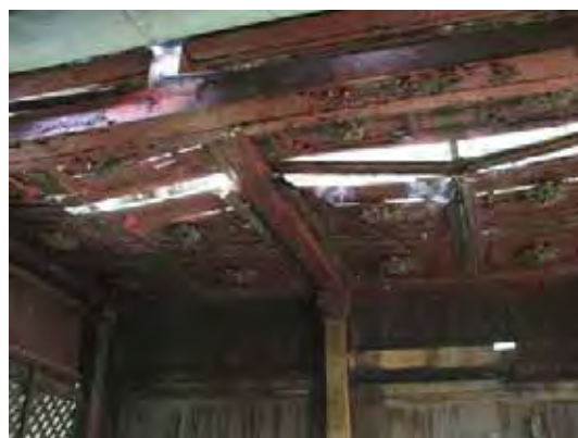
Figure 226: Condition of the ceiling. ( Photograph: 07.11.2008 )
