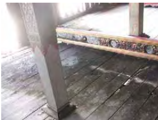
Figure 225: Condition of the floorboard. ( Photograph: 07.11.2008 )
