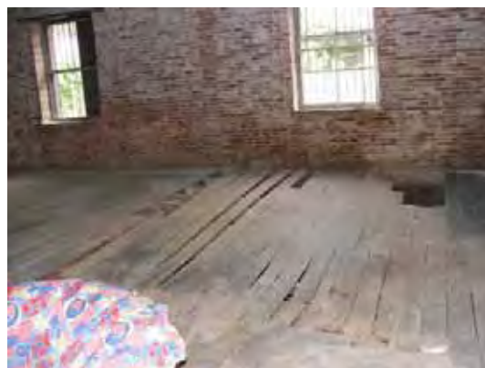
Figure 239: Incomplete floorboards at the non – living zone.
