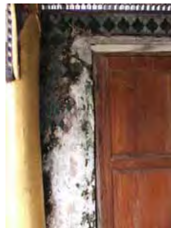
Figure 165: Efflorescence and lichen on the wall.
