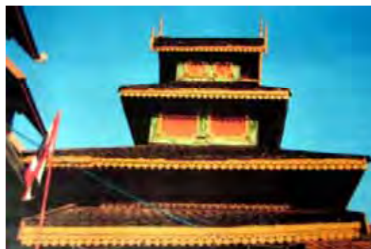
Figure 208: Condition of the tiered roof over staircase before restoration by Fine Arts Department. (Source: Fine Arts Department, 07.07.2009 )
