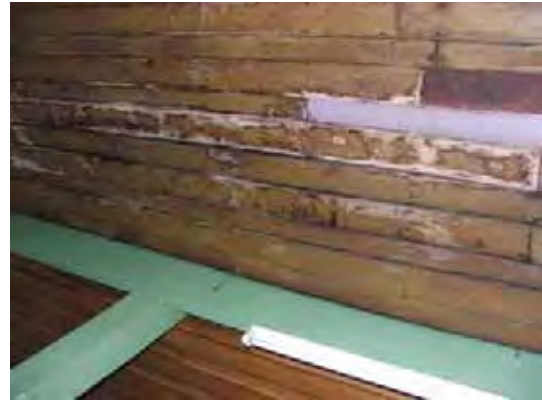
Figure 241: Leakage left its trace on wood ceiling.
