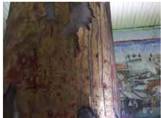
Figure 218: Peeled off pillar in the vihara. ( Photograph: 07.11.2008 )
