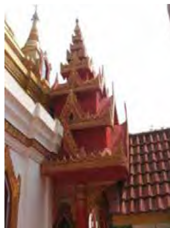
Figure 183: Condition of pyathat porch. ( Photograph: 19.02.2009 )
