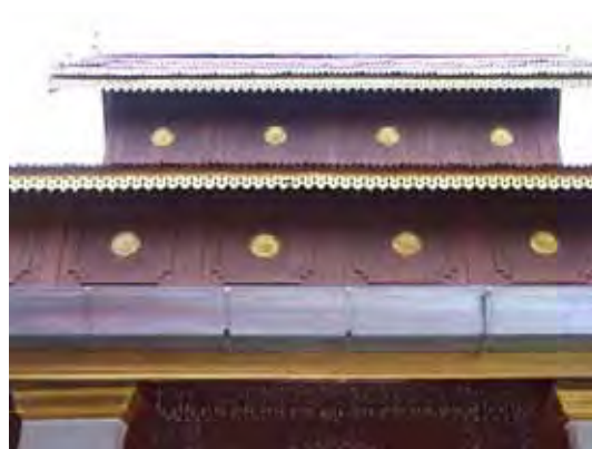
Figure 181: Condition of the upper part of the main hall. Notice the iron – sheet gutter.
