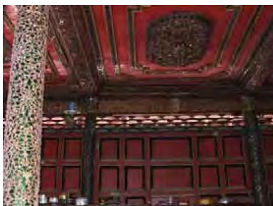
Figure 176: Condition of interior of the monastery. (Photograph: 17.11.2008)
