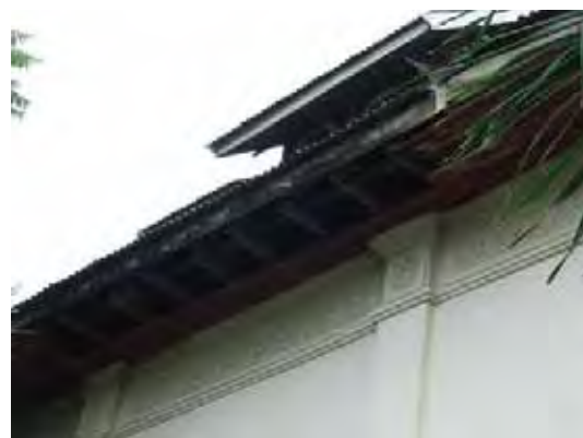
Figure 196: Terribly ruined at the eave.
