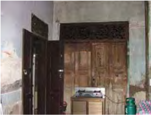
Figure 240: Efflorescent and fragment on the wall.
