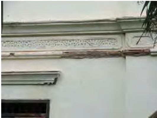
Figure 199: Ruined stucco reveals the structure.
