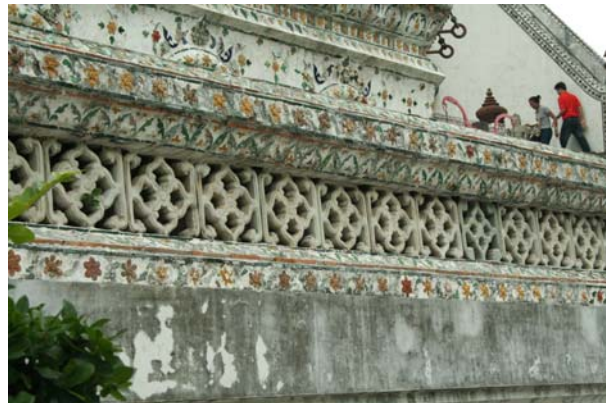
Figure 110: The wall of Phra Prang base showed sign of seepage by dampness causing decays
