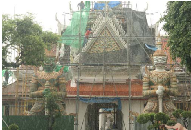
Figure 86: The restoration of the Entrance Way with Spire Roof in King Rama IX reign Photograph by: Kanjanaphorn Polprateep : May, 2008
