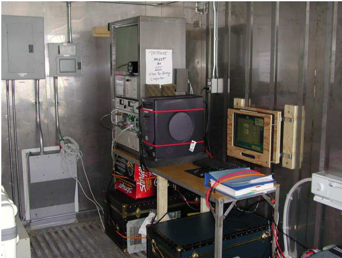
Figure 2.17: Electronics racks. Most of the electronics are located in the rack adjacent to the onboard computer.
