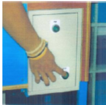
Fig. 6 Control box for the proposed module.
