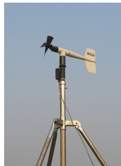
Figure 3.11. Wind monitoring device.
