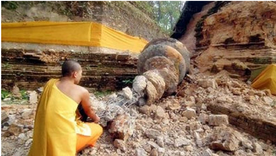
Fig. 39 Top of Chedi, heritage site in the northern of Thailand was collapsed from the earthquake on March 29th, 2011 reported by TTRWeekly newspaper
