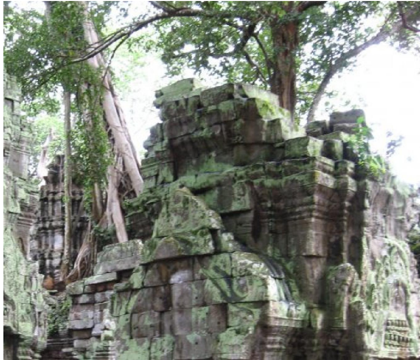
Fig. 41 The deterioration of the cultural heritage Prang as Buddhist Sanctuary Ta Prohm temple from root fig tree and lichen at the surface of the stone.
