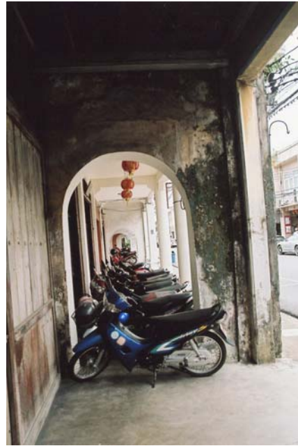
Figure 189: Humidity problems of the five-foot way of Arcade in the Old Phuket Town
