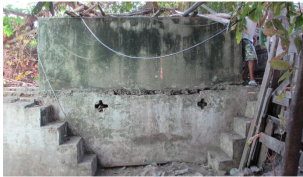
Figure 128 There were three layers of settlement wall used for protection. This is a second wall remaining after the outer wall collapsed into the river. Moreover, people brought bricks for their own proposes. Photograph by Phungwong, N. on October 21, 2011.
