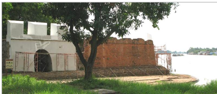
Figure 30 The remains of form Phom Phet (Diamond) or Phet Fort which protected the city from marine invasion and controlled ships coming from the sea. This fort is located in the southern part of Ayutthaya. The Fort was expanded and reinforced in European format in King Chakkraphat period (1548-1568). Photograph by Phungwong, N.
