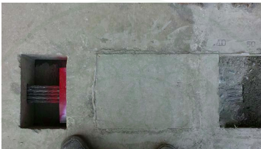
(a) The slips occurred during the time of cutting of concrete at step 50 cm to 40 cm.
