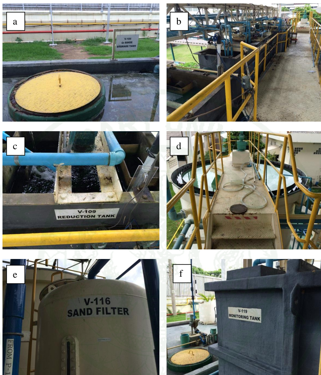
Appendix Figure C1 a) Rinsing chromium wastewater storage tank, b) Wastewater treatment units, c) Reduction tank, d) Sedimentation tank, e) Sand filter, f) Monitoring tank
