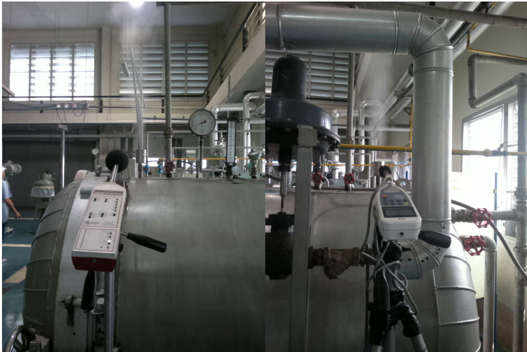
Figure A-8 The points of sound pressure level after install silencer for noise reduction testing from retort.
