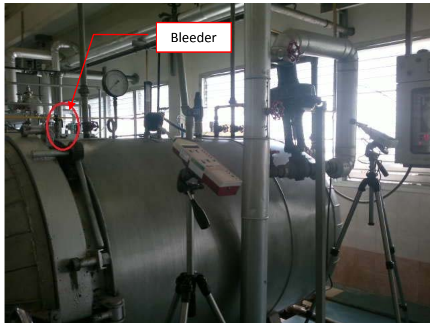
Figure A-6 The points of sound pressure level before install silencer for noise reduction testing from retort.
