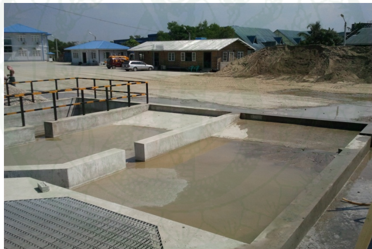
Figure 17 Sedimentation pond for process water
