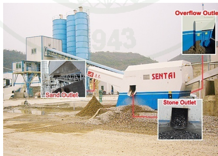
Figure 21 One of reclaimer unit in CBP of Yangon City
