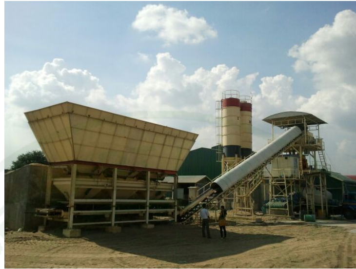
Figure 14 Enclosed system for hopper and conveyor for noise control
