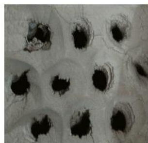
a) Dirty boiler fire tubes
