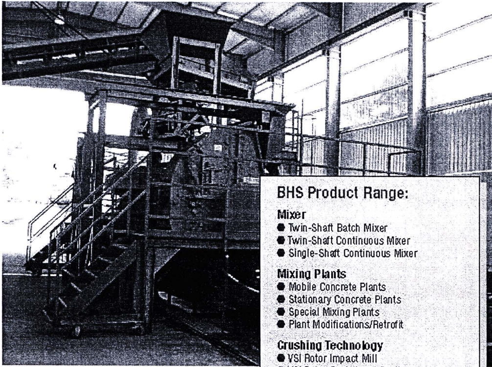
Crushing test centre in Sonthofen
