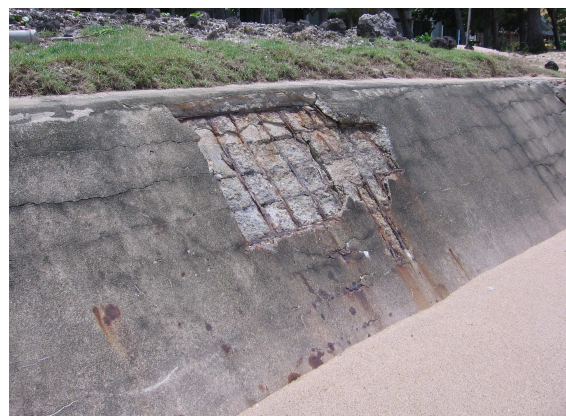
Figure 4-8 The seawall is damaged
