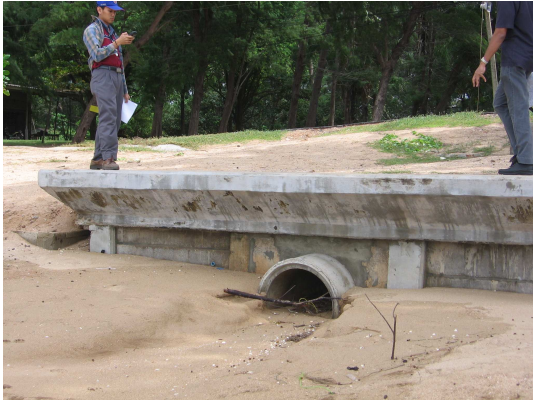
Figure 4-9 The seawall has to repair
