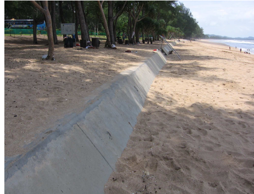
Figure 4-10 The seawall has to repair
