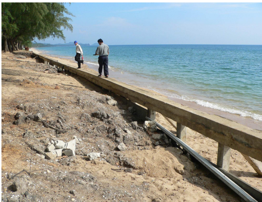
Figure 4-7 The seawall is damaged
