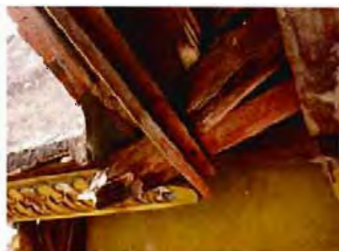
Figure 9: Under roof valley in decayed
