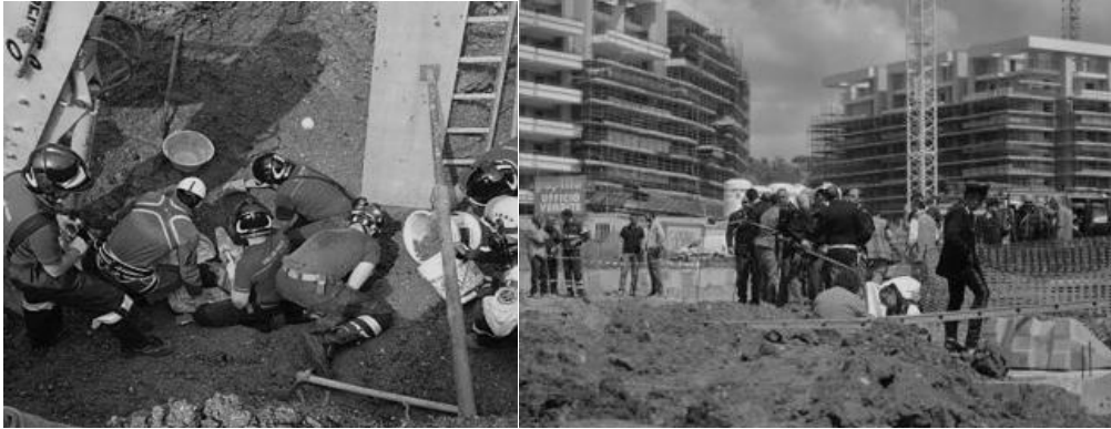
Figure 1. Excavations in the trenches. Incidents in the year 2014 on construction sites in Turin and Rome.
