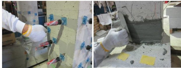
(a) Rebuilding of damage cross section with PCM (b) Injection of epoxy resin cross section with PCM
